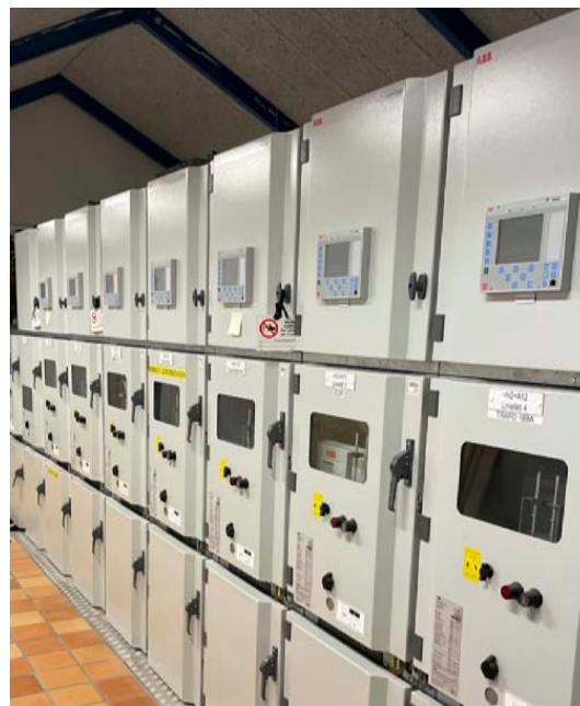
Ny 10 kV-afgang, station Nordhavn
